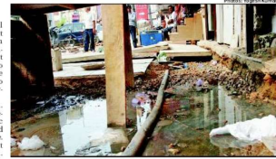
DANGER ZONE: Shopkeepers say many of them have fallen ill due to waterlogging and open drains.
